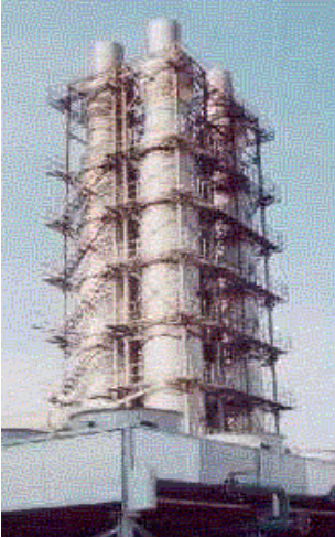
At Siirt Electric Power Plant, a KARE-Engineering Wet FGD is used to convert this 57,5 MW station into Clean Air Act compliance.
