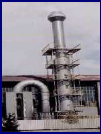
At Kayseri Orta Anadolu Mensucat Plant, a KARE-Engineering Wet FGD is used to bring this 21 MW station into Clean Air Act compliance.
