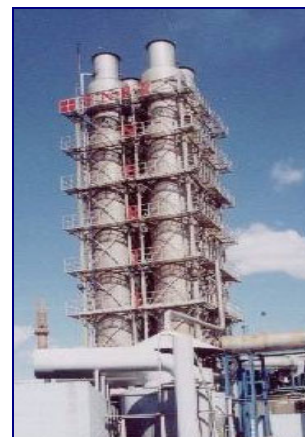
At Van (Ener Energy) Electric Power Plant, a KARE-Engineering Wet FGD is used to convert this 57,5 MW station into Clean Air Act compliance.
